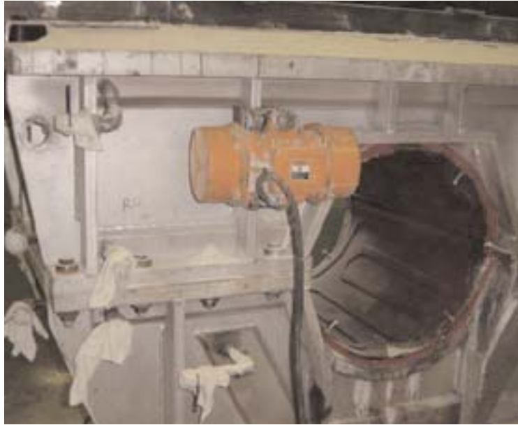
The EVS vibrator unit is seen here mounted to the inductor channel loop form.
