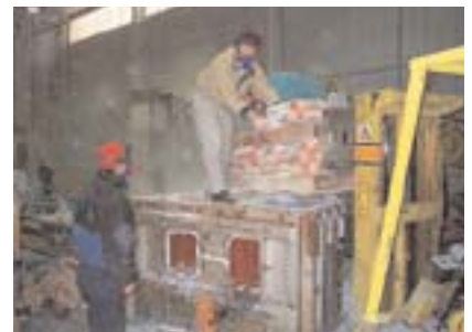
A view of the installation effort for dry vibratable refractories from bulk packaging.
